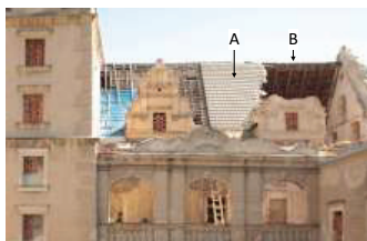
Fig. 1. Roof structure failure in the Gorzanow Palace
