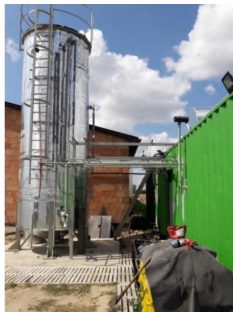
Photo 1. Pilot installation – examples of techniques of the anaerobic fermentation of waste – mono-substrate reactor (phot. G. Wałowski)
