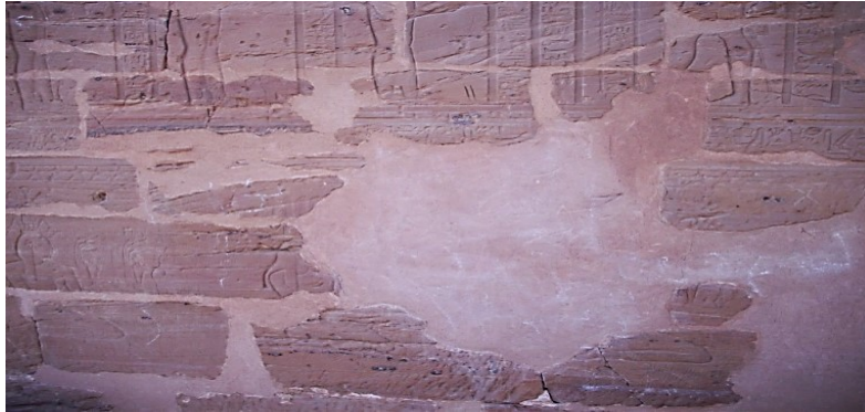
Fig. 11. The disappearance of the texts, symbols, inscriptions as a result of the deterioration caused by physical and chemical weathering
