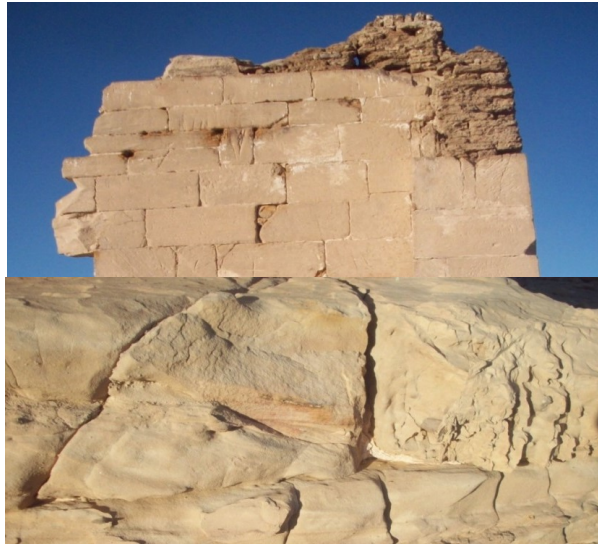
Fig. 4. A, B. Longitudinal single cracks on the wall of El-Nadira Temple, millimeters in width and centimeter in length, due to arid climate and wide range of temperatures.
