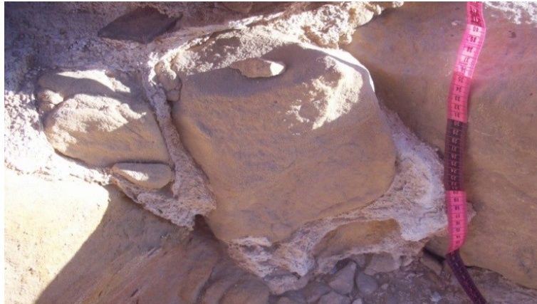
Fig. 13. Disintegration of the mortar used in jointing the stones wall at El-Nadora Temple as result of climate conditions
