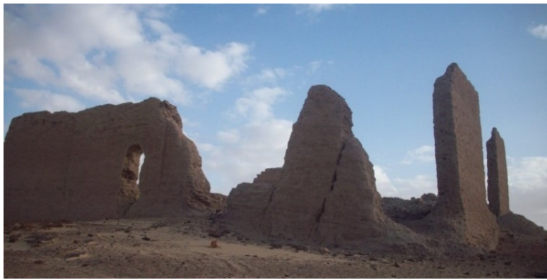
Fig. 9. The presence of structurally unstable walls at El-Nadora Temple as a result of physical weathering (natural causes), or constructional causes
