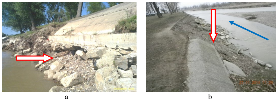
Fig. 9. Images of the protection works on the Moldova River: a - degraded left bank defence (2012); b - total left destroyed defence (year 2012) (Luca M., 2012).
