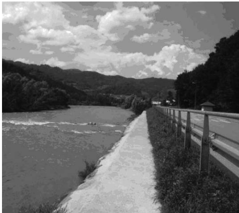
FIGURE 3. Concrete embankment as a strengthening of the right bank of the river – cross-section XI (km 19+870), (photo by M. Nawieśniak)
